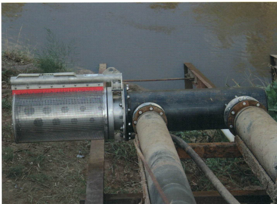
Cylinder screen on dual pipe.
